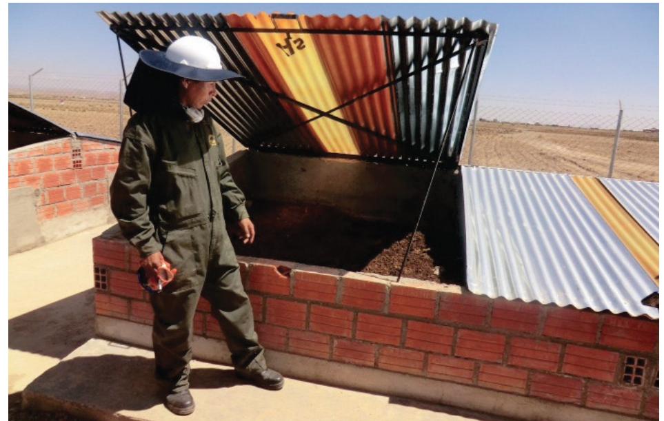
Huasi is vermi-composting faeces with subsequent solar drying in the same compartment in El Alto, Bolivia (Photo: H. Hoffmann, 2012).
